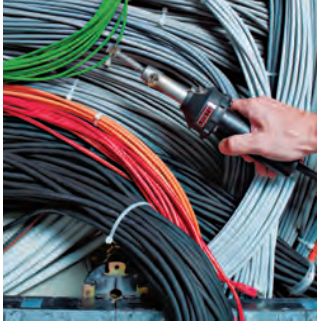
Fitting a solder shrink connection with HOT JET S and a push-fit sieve reflector.
